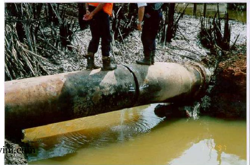
Pipe rupture location
